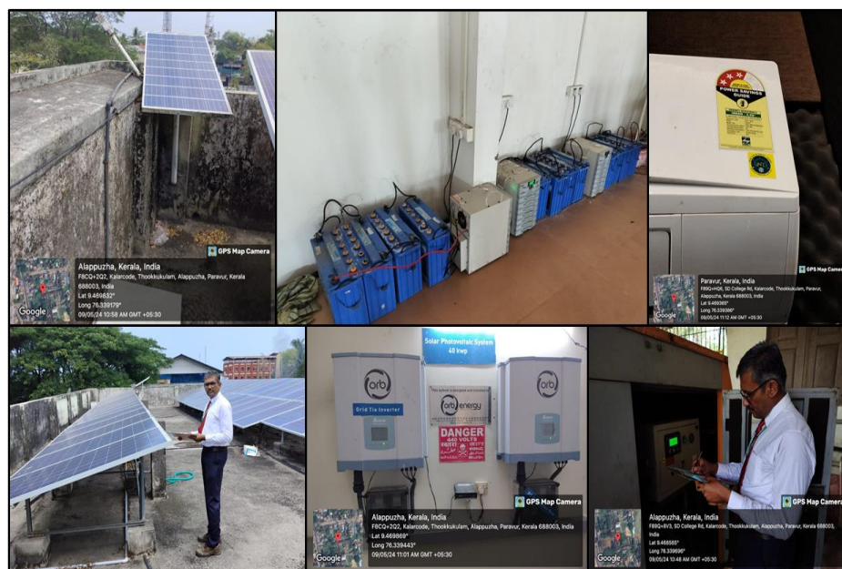
Energy conservation facilities observed in the Campus
