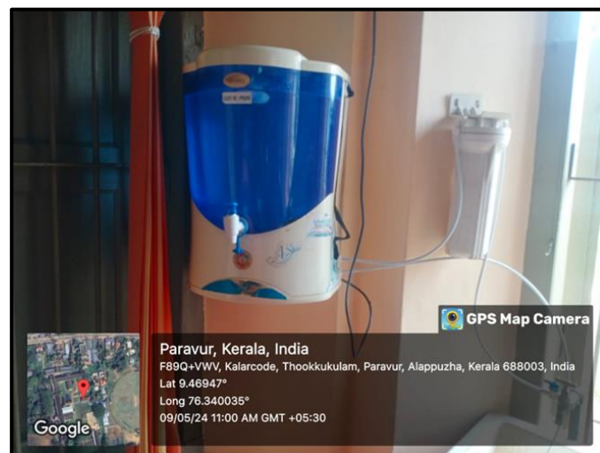
Drinking Water units observed in the campus
